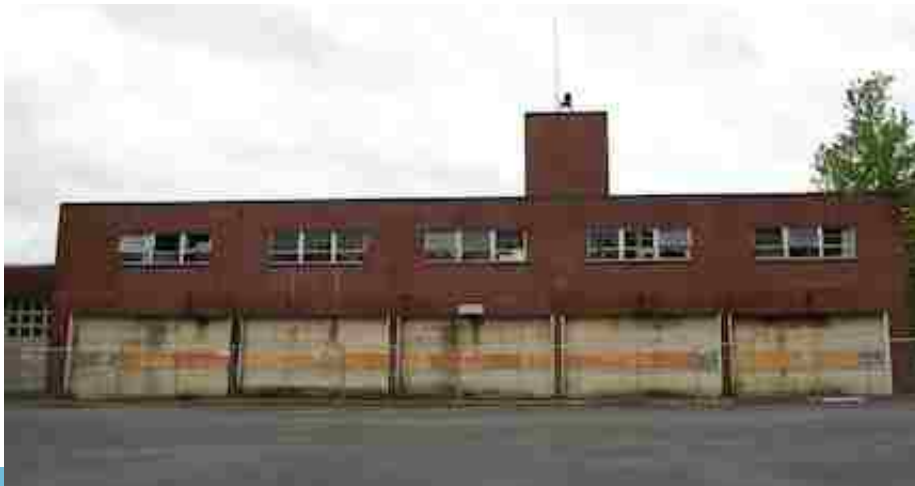
Figure 33. North side of Building 18 in 2009, Photography by Artifacts Consulting, Inc., 2009. Source: Sally Bagshaw, Blog Archive, Parks
