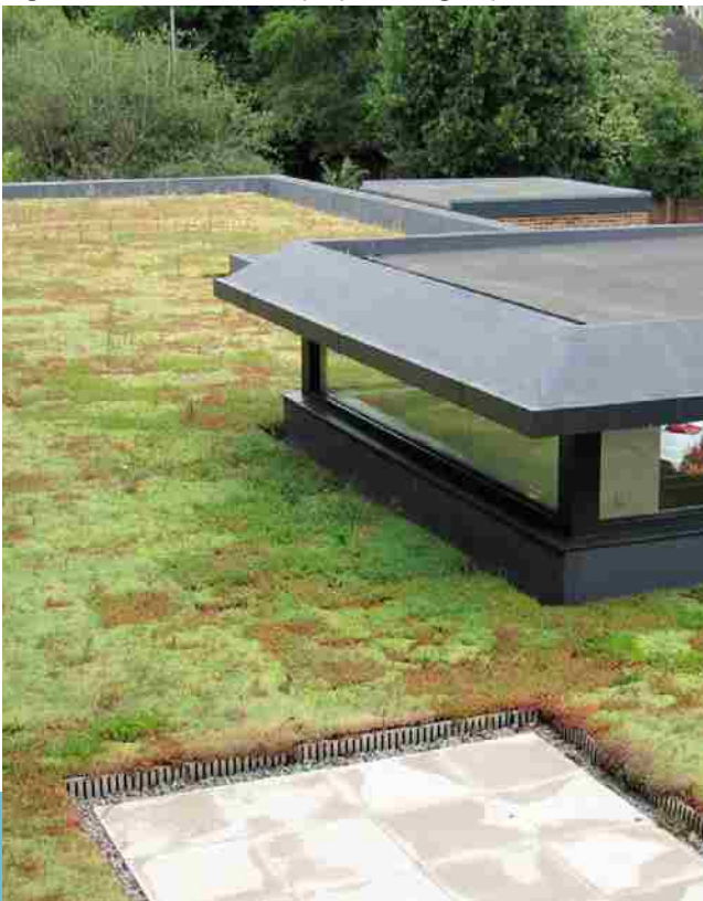
Figure 93. Sedum Rooftop by Roofing Superstore
